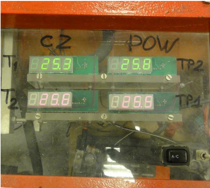
Fig.19. Panel of the stand with temperature gage and A/C switcher
